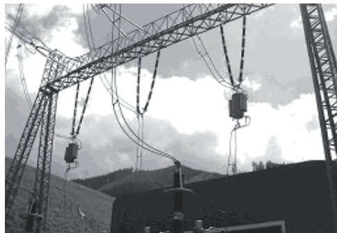
Ryc. 4. Leading out of the capacity from the station
